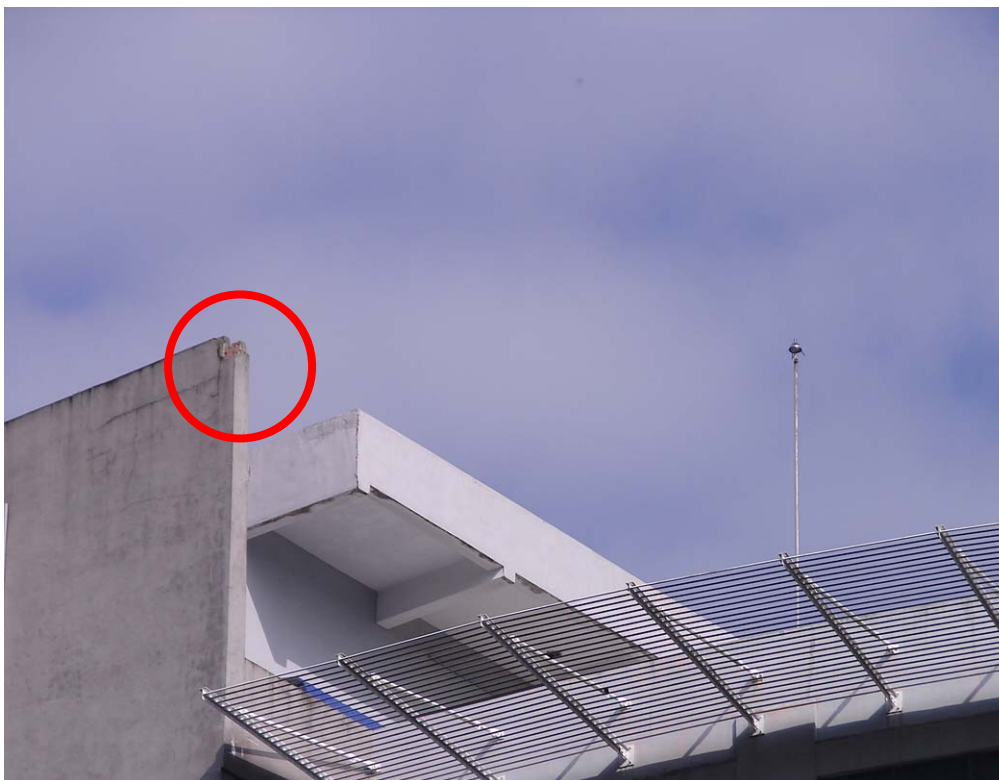
Fig. 13: The lightning damaged TNB building in Johor Baru, Malaysia.
