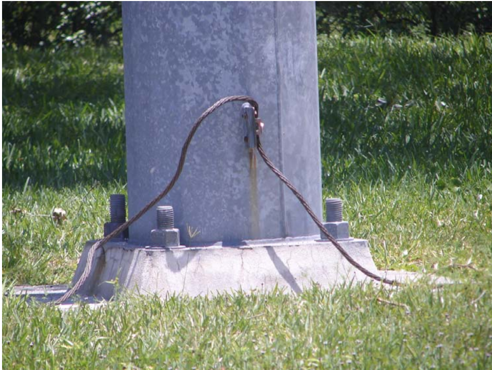
Fig. 7: The base of the ESE lightning rod mast at B showing a grounding cable leading towards two grounding points..
