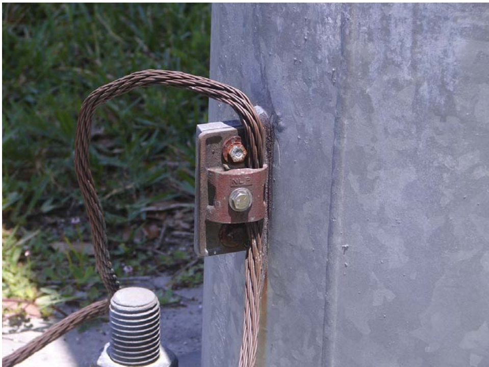
Fig. 8: A close-up shot of the bonding terminal on the mast..
