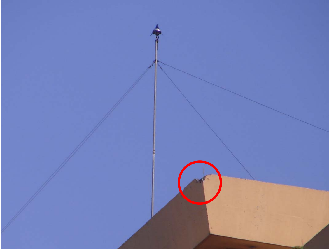
Fig. 14: The lightning damaged Sri Kota apartment in Kuala Lumpur, Malaysia.
